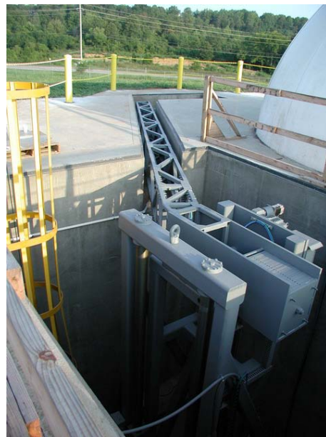
Figure 3. Theta Positioner Installed in Pit
